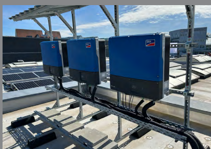
PV-Anlage in Bayreuth
